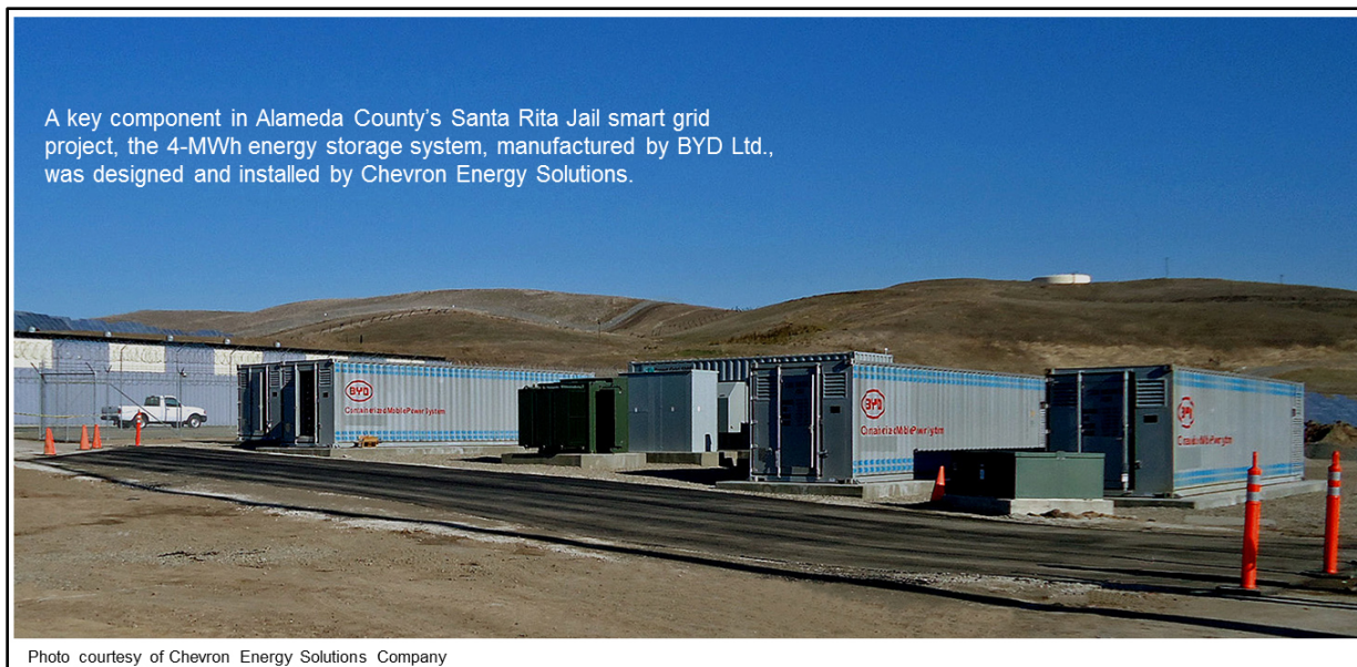
Figure 98. A 2-MW/4-MWh Li-ion Energy Storage System
