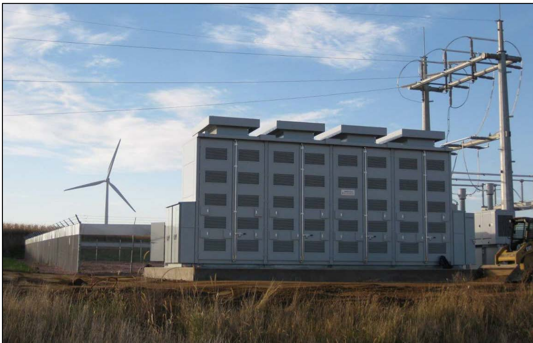
Figure 34. Xcel Battery Supplementing Wind Turbines, Lucerne, MN
