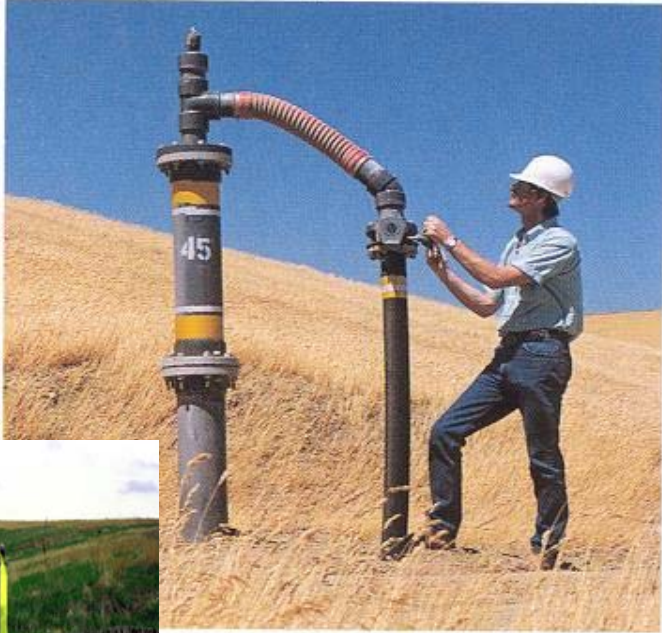
A typical gas recovery well
