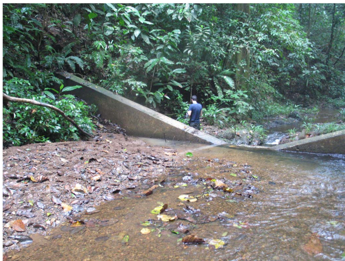
Fig. 2. Fully sedimented forest catchment weir in Soberania National Park, Panama, provided the impetus for this study (weir location: 9^{\circ} 12' 32'' N, 79^{\circ} 46' 46'' W) (image by Fred L. Ogden)
