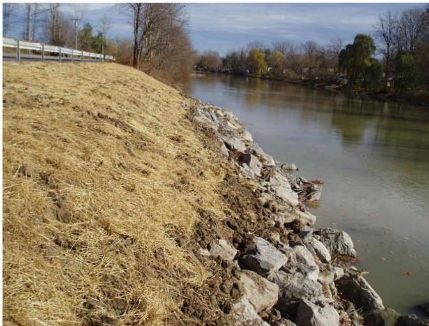
FIG. 21 STONE FILLING (HEAVY) INSTALLED AS TOE PROTECTION WHILE GRADATIONS IN UPPER PORTION OF SLOPE VARY IN LAYERS TO ALLOW TOPSOIL AND SEED
