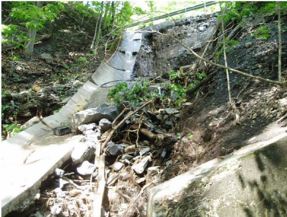
FIG. 23 FAILURE OF PORTLAND CEMENT CONCRETE CHANNEL LINING
