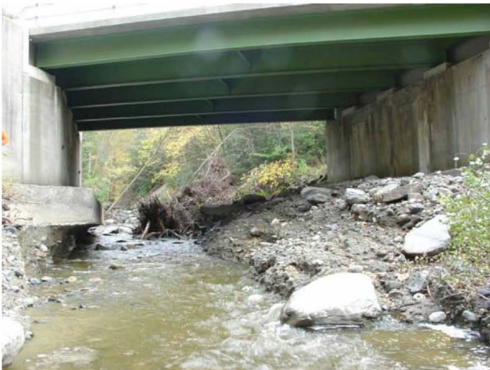
FIG. 2 CHANNEL BEND IN BACKGROUND DEFLECTS FLOW TOWARDS BRIDGE ABUTMENT AND UNDERMINES FOOTING.
