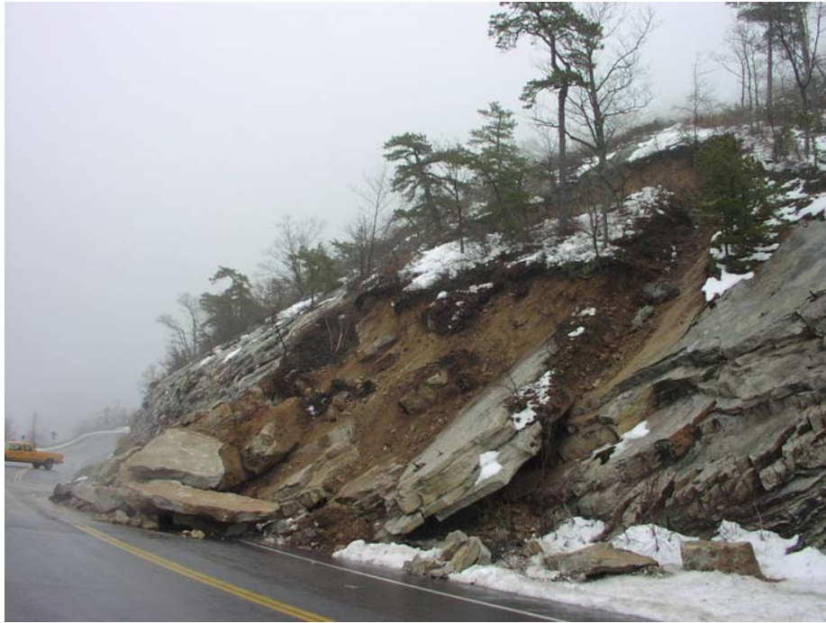
Figure 9-28 Large Scale Rock Fall
