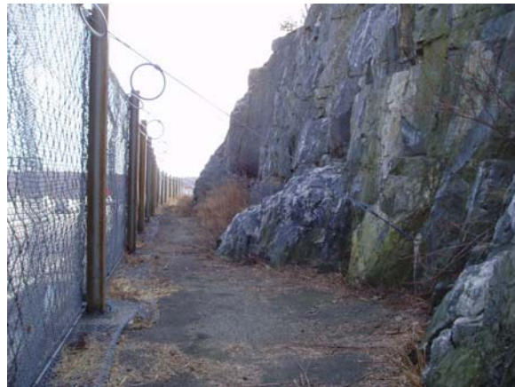
Figure 9-32o Wire Rope Catchment Fence (Medium Impact)
