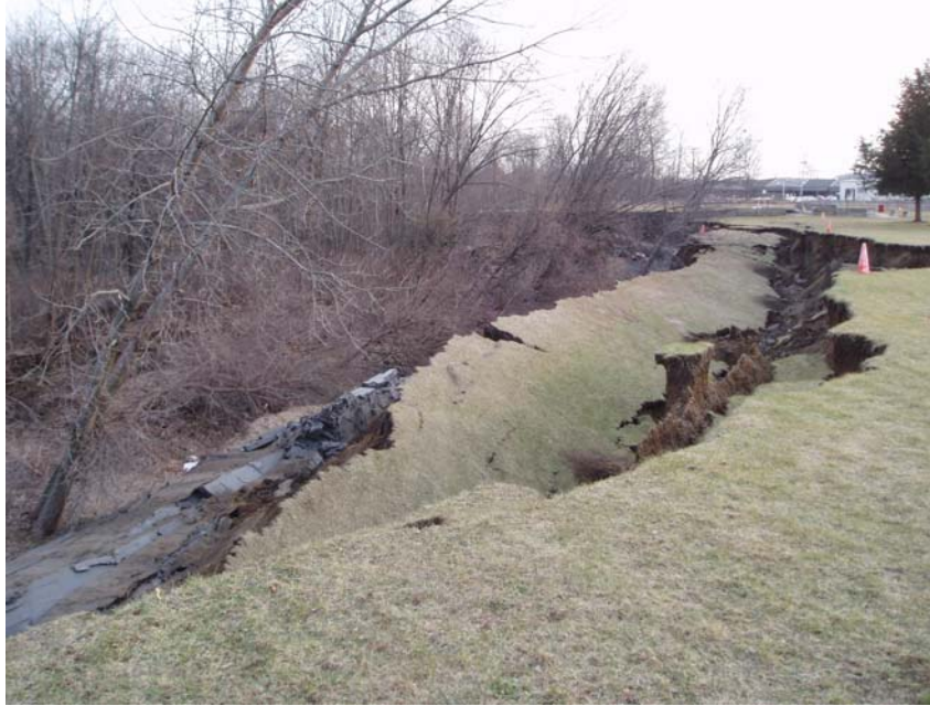
Figure 9-17 Deep-Seated Slope Failure
