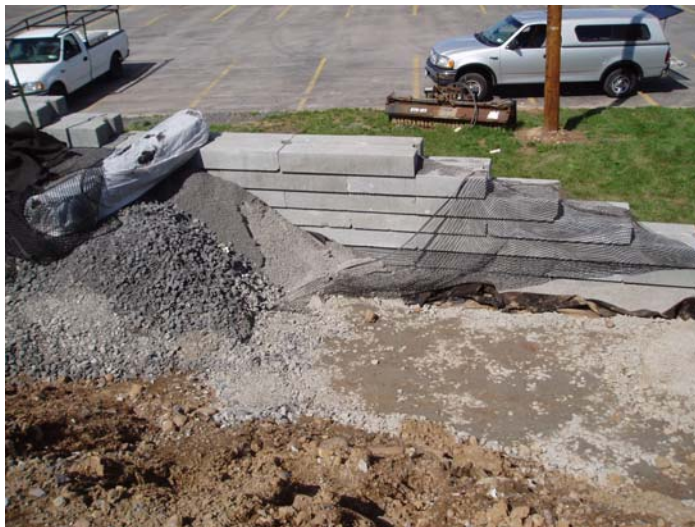
Figure 9-52b Mechanically Stabilized Segmental Block Wall System (Back Face) (Unilock Siena Stone 500 & Strata grid 200)
