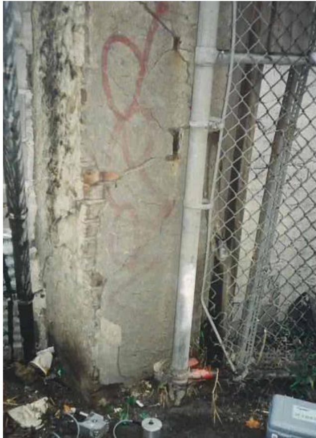
Figure 9-60 Vibration Monitoring of Adjacent “Suspect” Building
