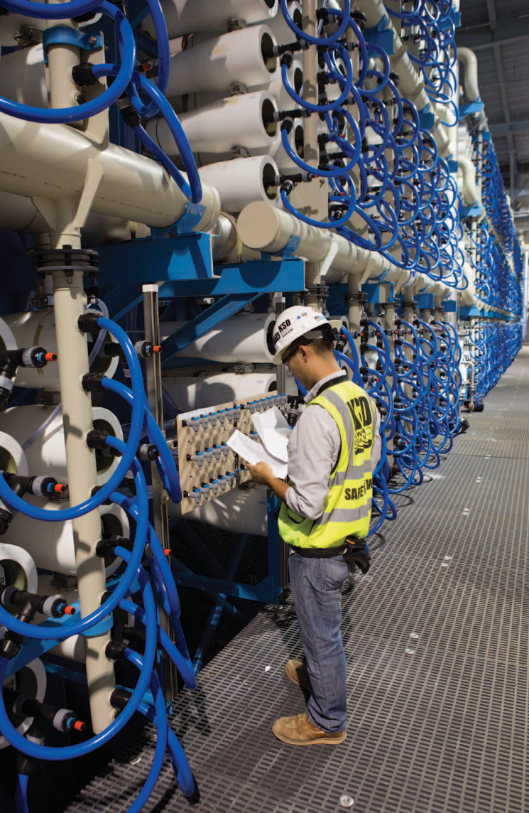
Pressure vessels containing reverse osmosis membranes are the heart of the Carlsbad Desalination Plant, to start supplying 8 percent of San Diego County with desalinated ocean water by mid-2016. Photo: Poseidon Water
